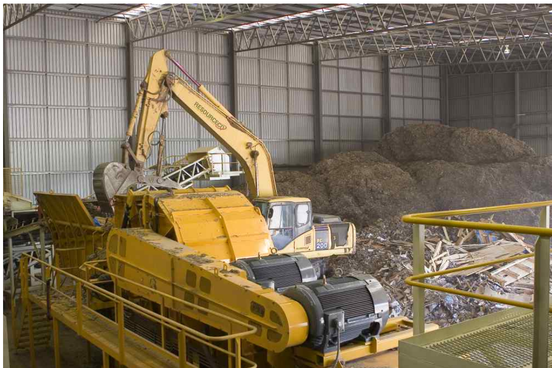
Alternative Fuel Processing facility Wilkins Road Gilman, This is a joint venture of Resourceco and Adelaide Brighton Limited.
