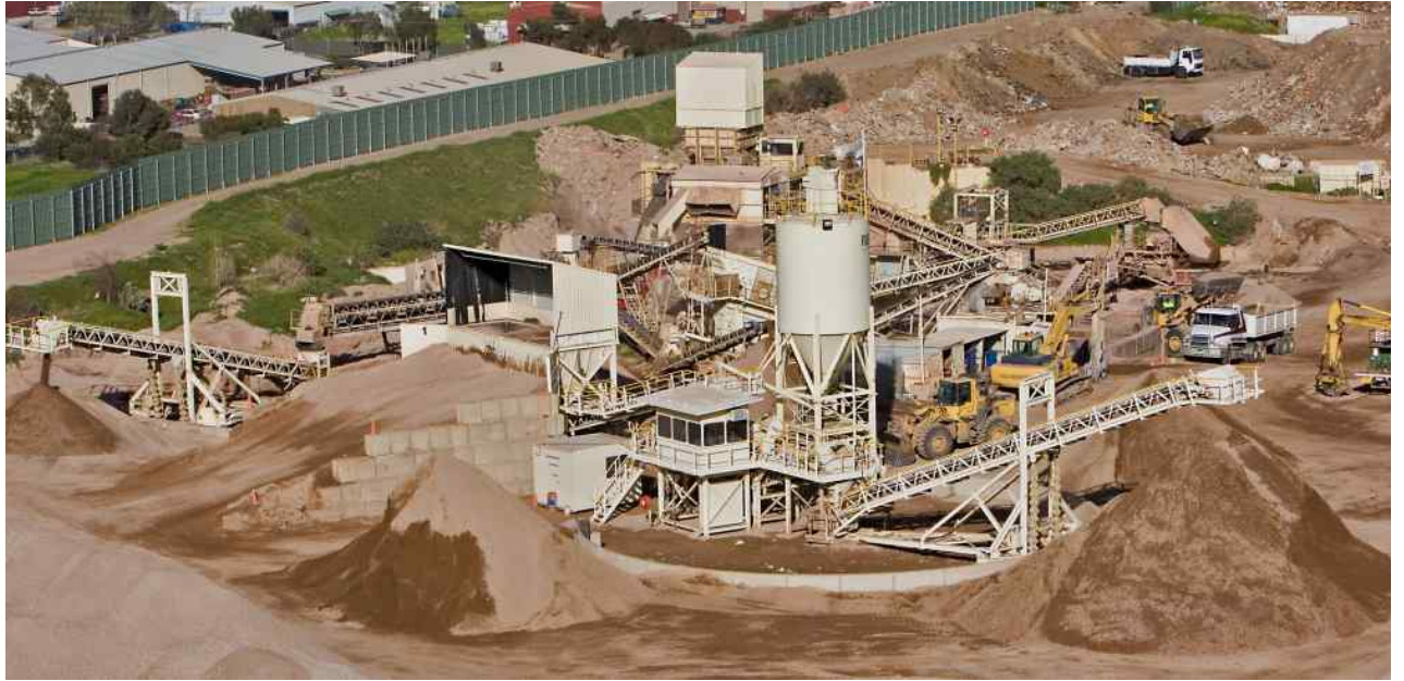
Resourceco Wingfield Crushing Circuit
